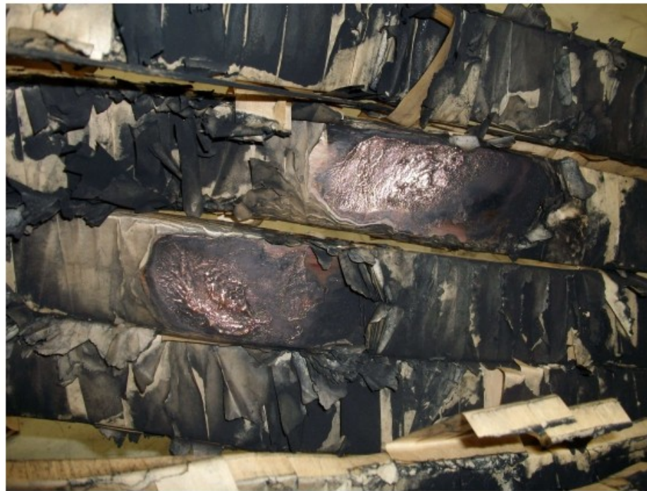
Fig 6. failure area , conductors „A“ and „D“ , second turn, inner layer
